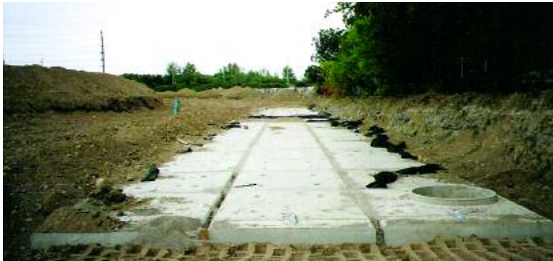
Tanks installed with access holes for man entry and maintenance and flow equalizers between each run of boxes.
