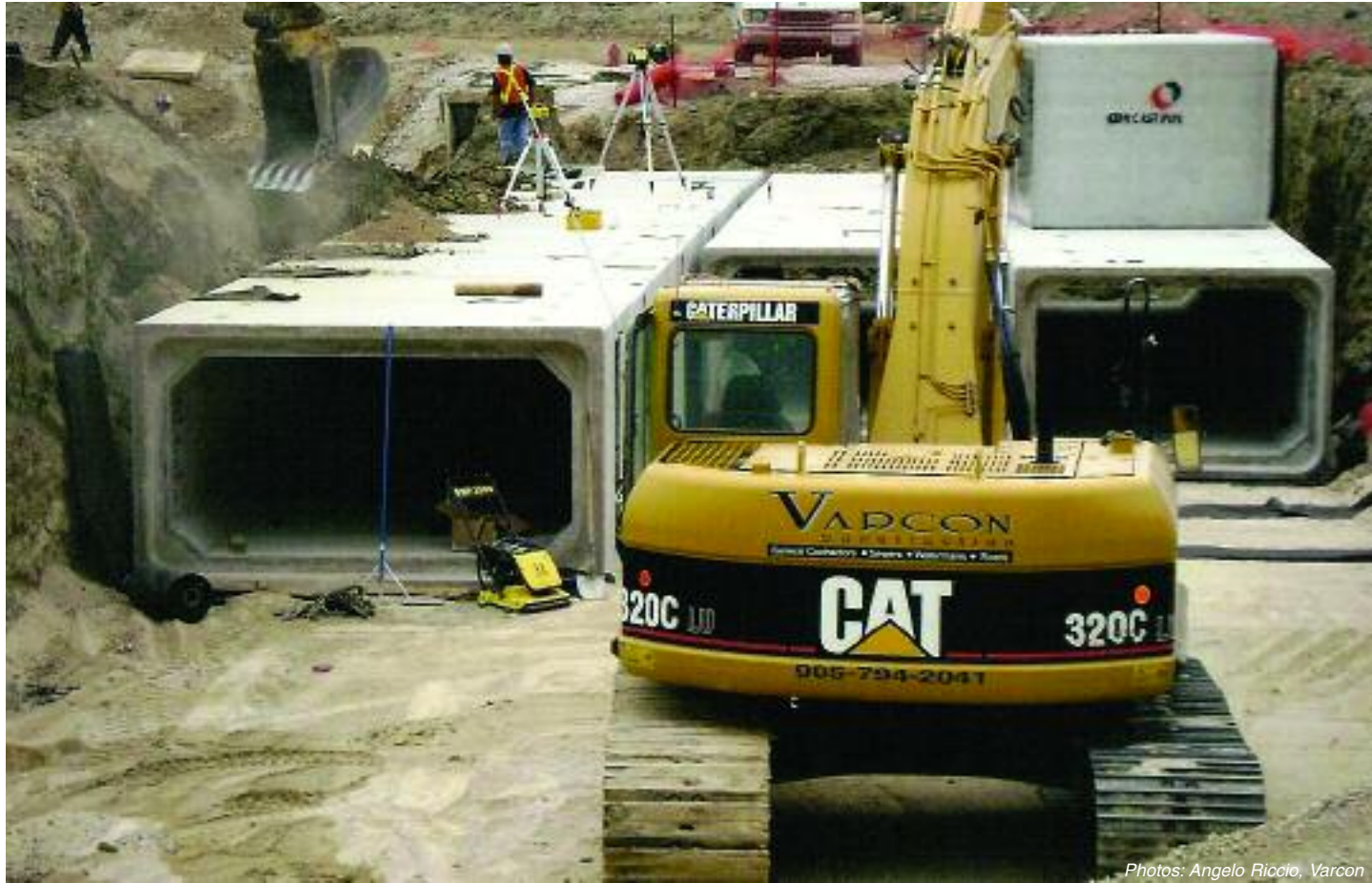
Photos: Angelo Riccio, Varcon Precast boxes required for construction of triple-celled storage tanks for storm water management.
